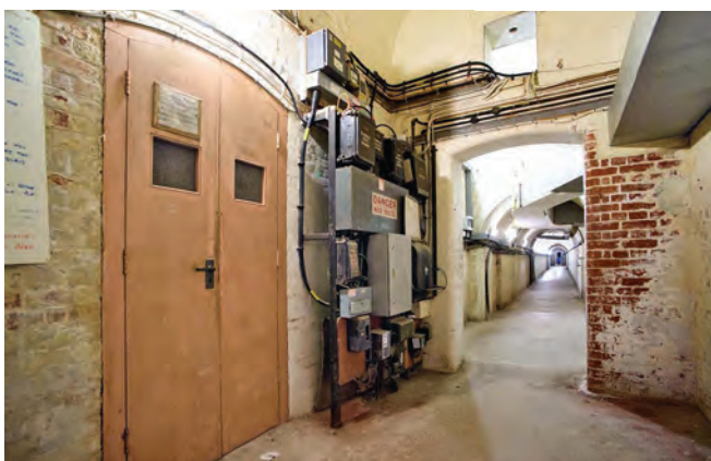
The tunnel from outside the entrance to the control centre at Fort Widley. Note the switchgear on the left.
